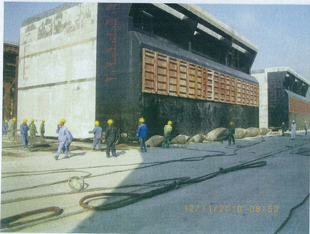
Photo record of SHK Centre Pumping Station (Great Eagle centre/ Harbour Centre Pumping Station, China Resources Building Pumping Station similar)
